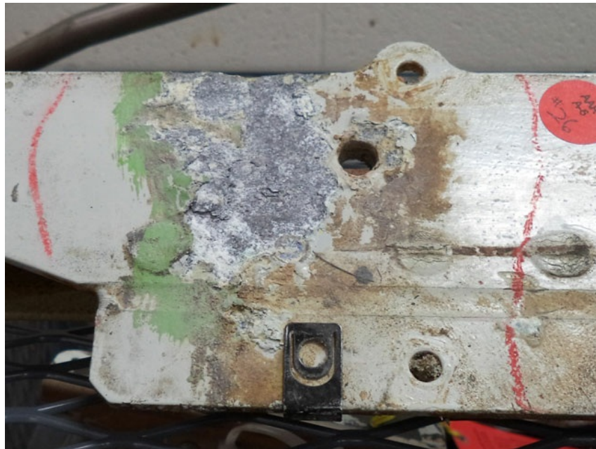
Corrosion on Structure Beam
