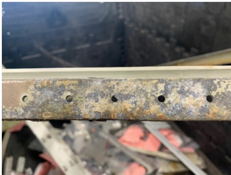
Corrosion on a beam
